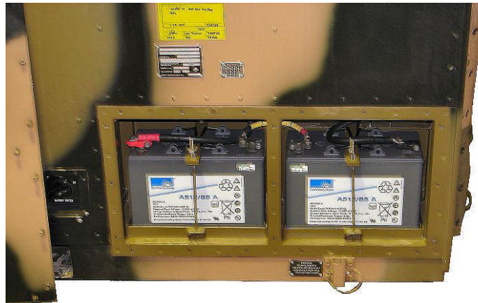
Figure 113K-6: Circuit Switch Assemblage Battery Bay
