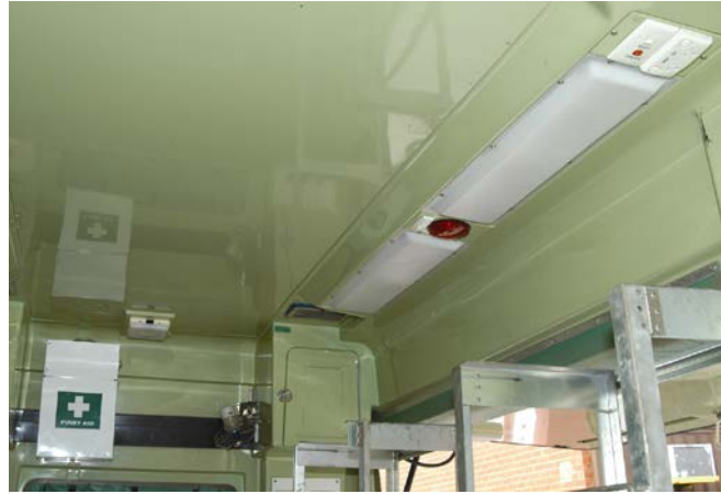
Figure 113D–5: General Maintenance Vehicle Repair Module Interior Lights
