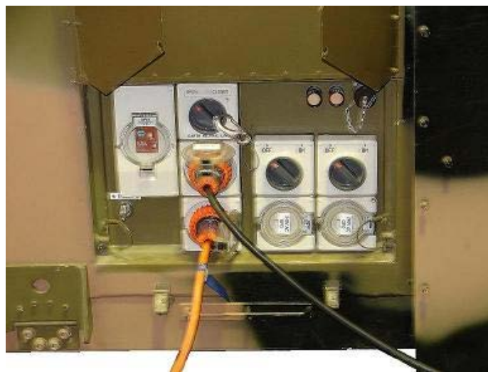
Figure 113K-7: Circuit Switch Assemblage External Power Access Cover
