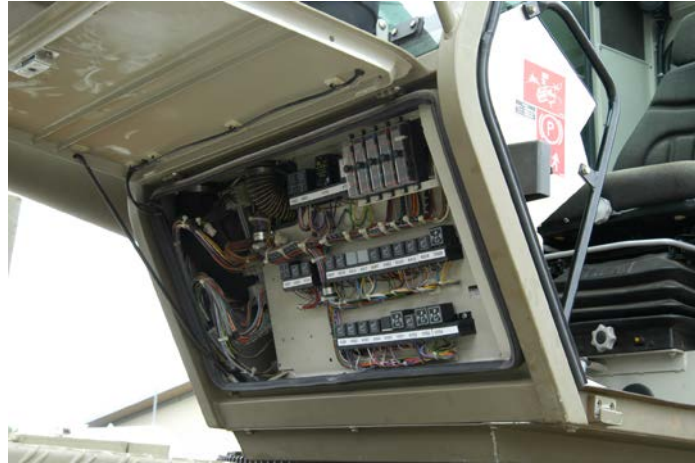
Figure 32A–30: Tadano’s Crane Cab Instrument Electrical Fuse Panel
