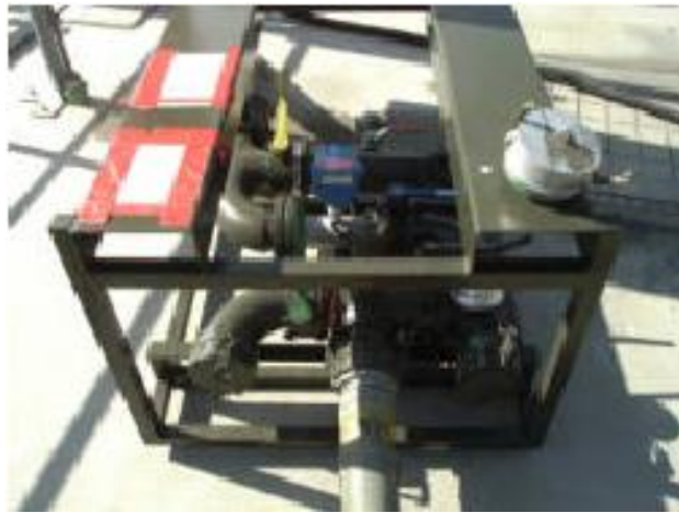
Figure 33C–2: Tank, Fabric Collapsible Marine (TFCM) Meter Manifold
