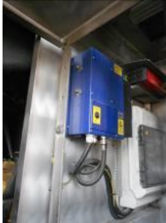
Figure 47A-9: Panther’s electrical boxes
