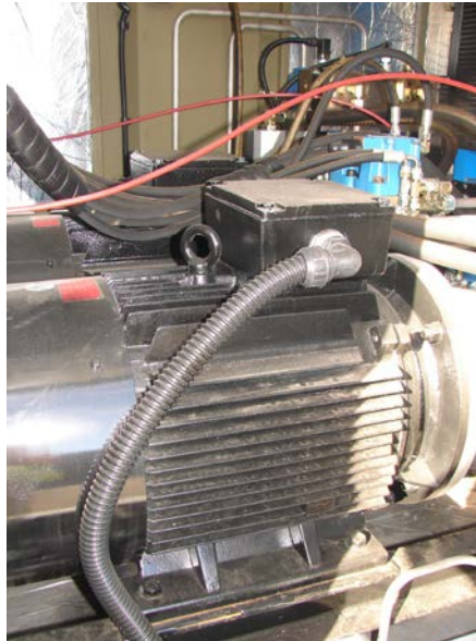
Figure 49D-11: Berendsen 10 GPM Hydraulic Unit's Hydraulics
