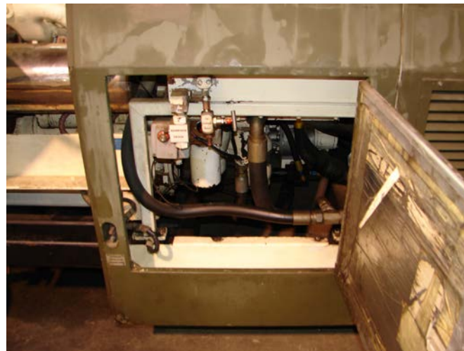
Figure 49C-6: Rexroth 35 GPM Hydraulic Unit's Hydraulics
