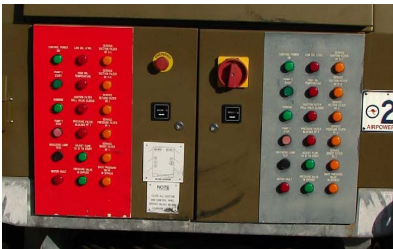
Figure 49D-5: Berendsen 10 GPM Hydraulic Rig's Dual Pump Control Panel
