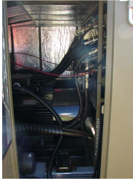
Figure 49D-10: Berendsen 10 GPM Hydraulic Unit's Hydraulics
