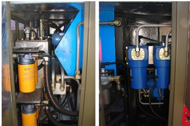
Figure 49D-8: Berendsen 10 GPM Hydraulic Unit's Engine Bay
