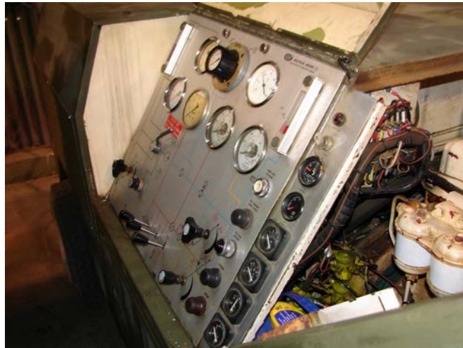
Figure 49C-3: Rexroth 35GPM Hydraulic Rig Unit's Control Panel
