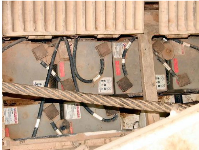
Figure 90–45: M88A2 Hercules HRV's Battery Bay
